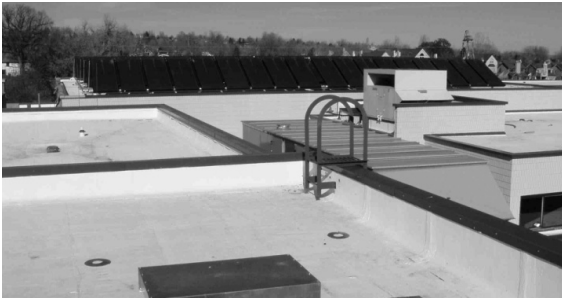
Figure 7. A modified bitumen cool roof with a white reflective coating was installed on the flat sections of the building's roof.
