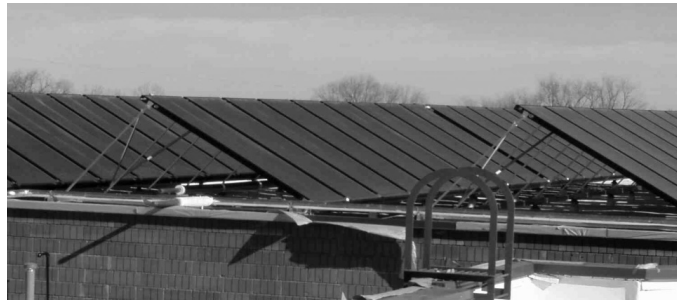
Figure 8. The North Boulder Recreation Center uses 557 m 2 of solar panels to pre-heat the water for the center's two swimming pools.
