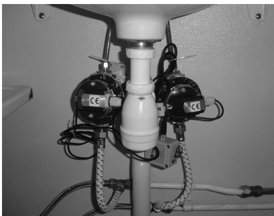
Figure 2. Two Macnaught flow meters mounted on the cold and hot water pipes below a basin.
