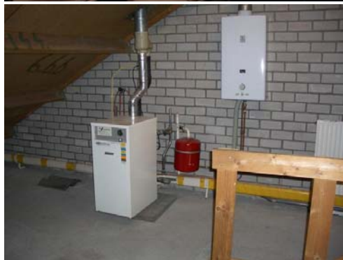
Figure 6-8. Boiler plus instantaneous gas water heater in loft [anonymous]
