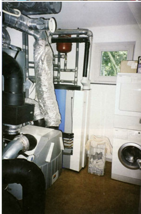
Figure 6-3. Gas storage boiler (together with central ventilation air heat recovery unit) in basement (Source: www.passiefhuis.nl )
