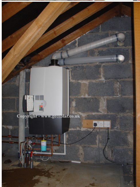
Figure 6-6. Boiler in attic [www.geosolar.co.uk]
