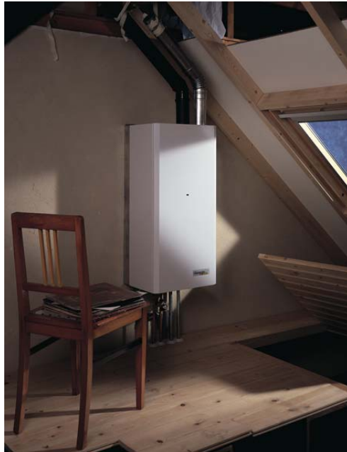
Figure 6-7. Boiler in loft [ www.vanderschaftbv.nl/htm/home.htm ]
