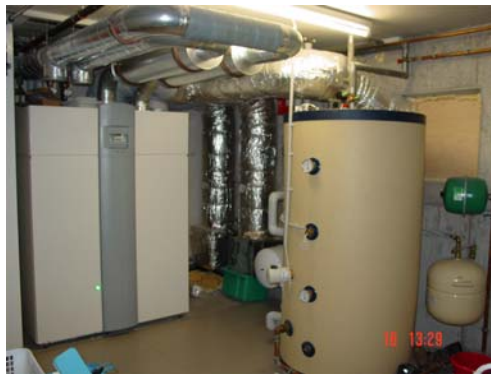
Figure 6-2. Heat pump in boiler room (Source: http://www.alfredschneider.de )
