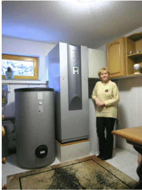
Figure 6-1. Heat pump in basement (storage left) (Source: http://www.waermepumpentag.de )
