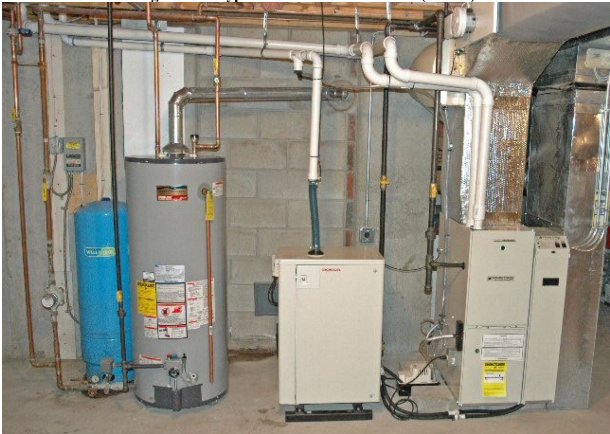
Figure 2. A Typical Field Test Installation (Site #6)
