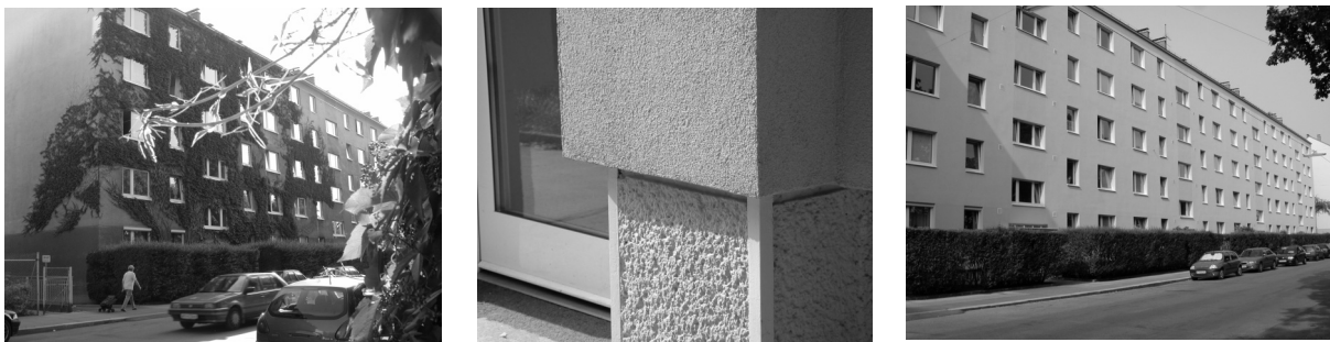
Figure 3: Pictures of the building before renovation (left), after renovation (right), detail of insulation application (middle)
