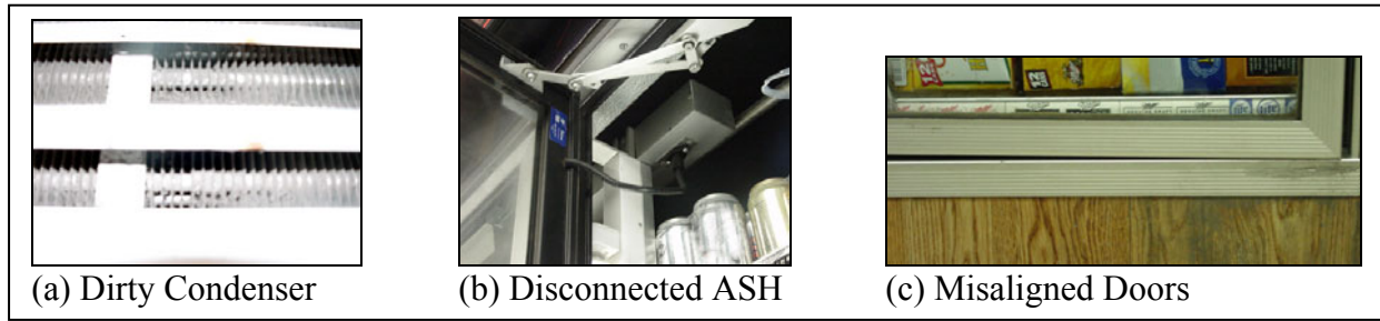
Figure 2. Samples of Neglected Maintenance
