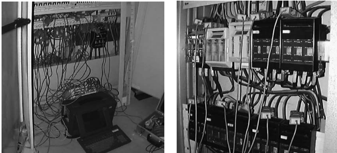
Figure 4. Multi Channel Load Monitoring in industry. Set up of measurement devices.
