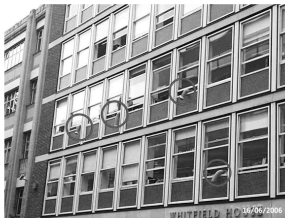
Figure 4. Hot air exhaust tubes or outdoor units.
